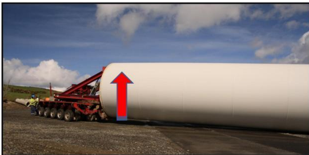
Fig. 13. Hydraulically adjustable trailer can elevate the rear clamp set of tower section
