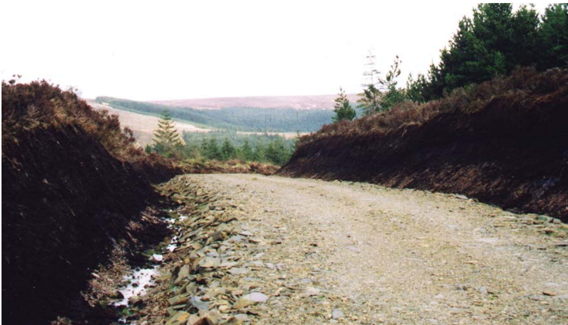
PHOTO 4: Forest road cutting.
